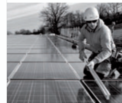
Nearly 1700 m 2 of photovoltaic panels on the roof of the new HEQ plant
